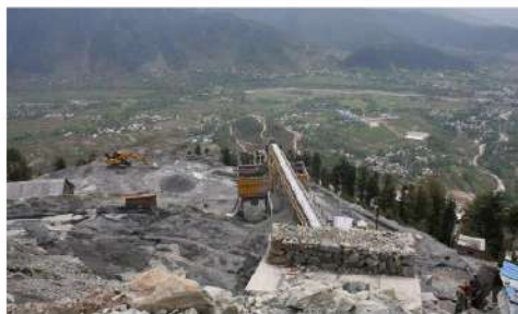
Work in progress on the Kishen Ganga Hydro Electric Power Project in North Kashmir district of Bandipora in 2012. NISSAR AHMAD
