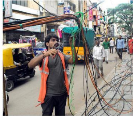
Major hazard: Officials remove Optical Fibre Cables which were hanging in Bengaluru, 2018. FILE PHOTO
